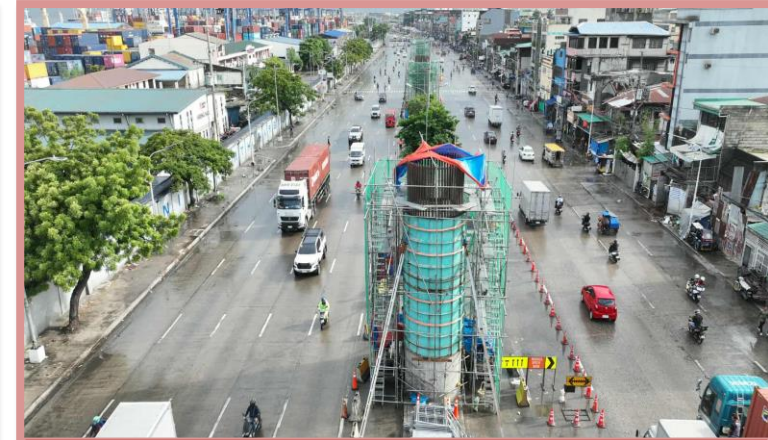
SP-53: Ongoing rebar installation in preparation of casting column for 2 nd lift
